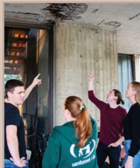
The concrete falling from the roof outside of Aud.Max. can create dangerous situations for the students.
